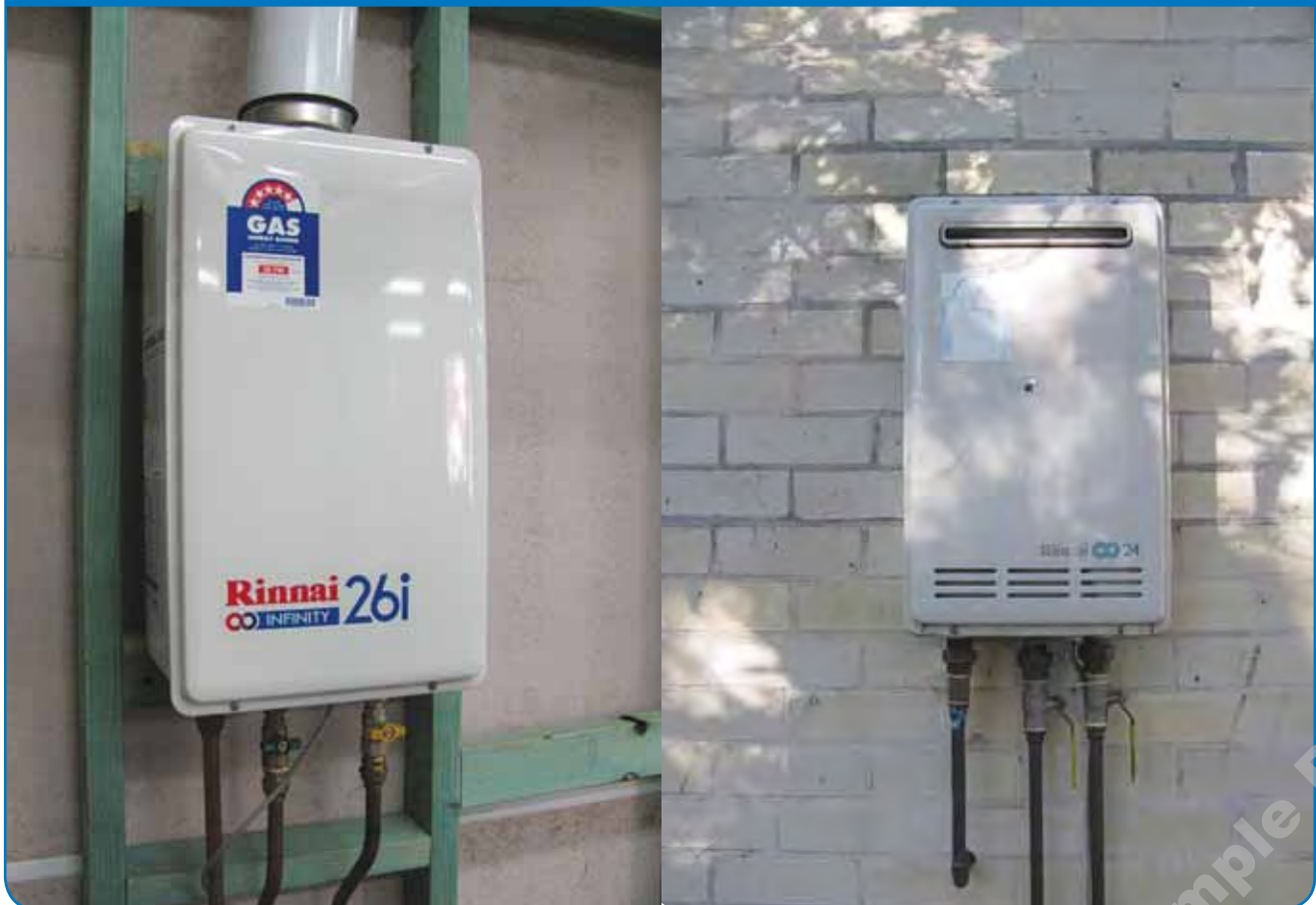
FIG 11.15 (a) Continuous flow hot water service (interior) and (b) exterior
